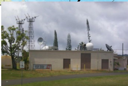
Hawaii USCG COMSTA 2 LEO/MEOLUT & 6 antenna MEOLUT Refresh and Phased array funded by NOAA underway
