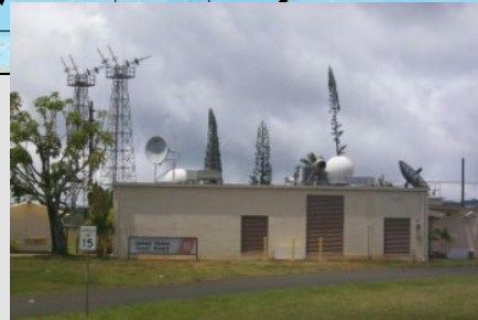
Hawaii USCG COMSTA 2 LEO/MEOLUT & 6 antenna MEOLUT Refresh and Phased Array Antenna planned
