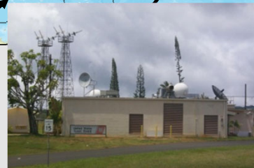
Hawaii USCG COMSTA 2 LEO/MEOLUT & 6 antenna MEOLUT Refresh and Phased array funded by NOAA underway (FAT in California)
